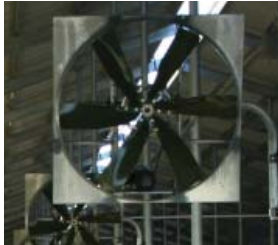
Fans must be in proper condition to cool cows.
