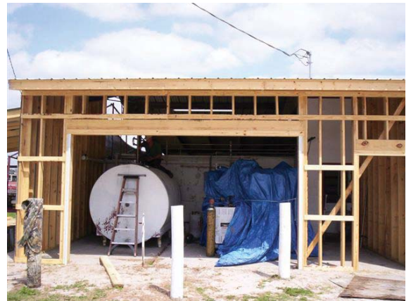
A look at the pasteurizer being put into place. Photo by Rick Hedrick.
