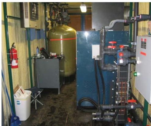
A look at the system at DPS - Georgia.
